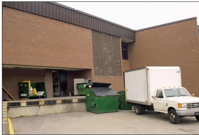
Photo 1: Truck exhaust and odors entered the building at the school's loading dock.
