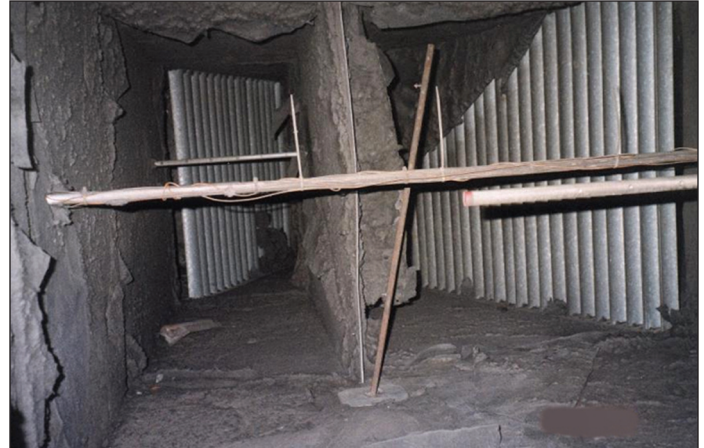
Photo 2: The high velocity, turbulent airstream severely damaged interior fibrous glass insulation just downstream of the supply fan's blast zone.
