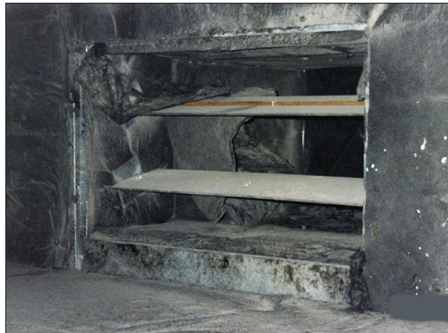
Photo 3: Large sections of the interior fibrous glass insulation had released from the metal ductwork, becoming lodged in balancing dampers.
