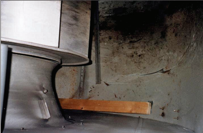
Photo 1: A length of angle iron and a section of lumber were found in the scroll of the supply air fan. Apparently, both had been there since the time of original construction.
